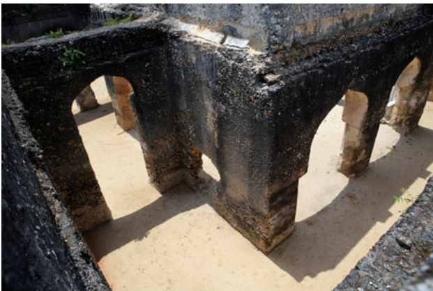
14.12 The arcades around the central inner court of the Mtoni Palace. Photo Mieke Woestenburg
