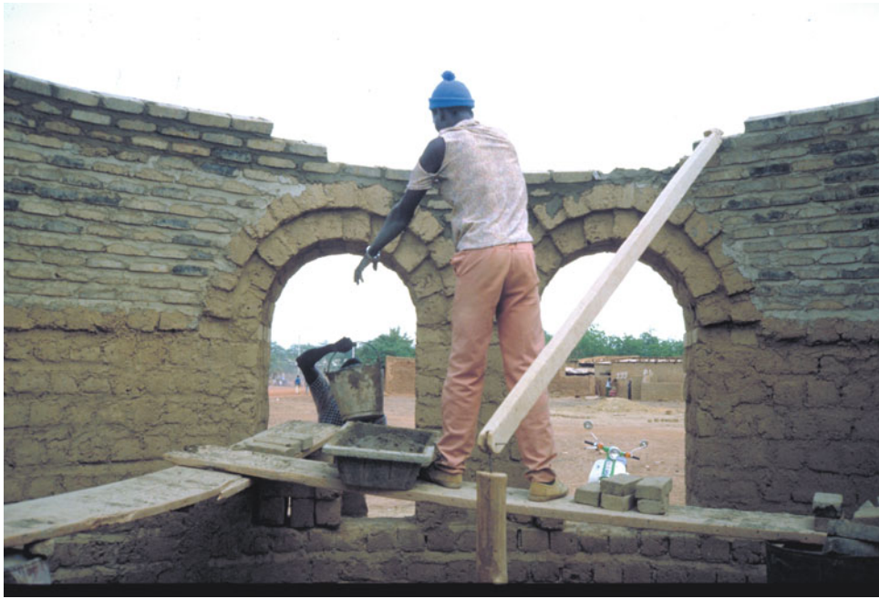
8.15 The construction of the DGUT field office cupola without use of formwork
