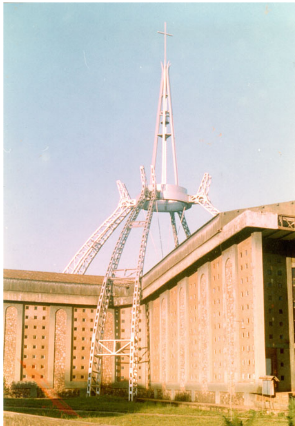
17.5 The Mater Misericordia in 1991. The covering of the flying buttresses has completely disappeared and the roof is in a bad state
