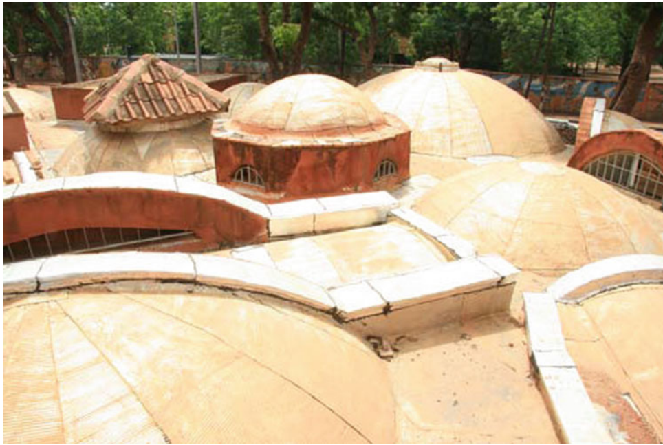
9.1 The Centre Matériaux in Ouagadougou in 2008. All openings are closed and the roofscape is covered with all sorts of sealants, paints, and flashings. Photo Belinda van Buiten
