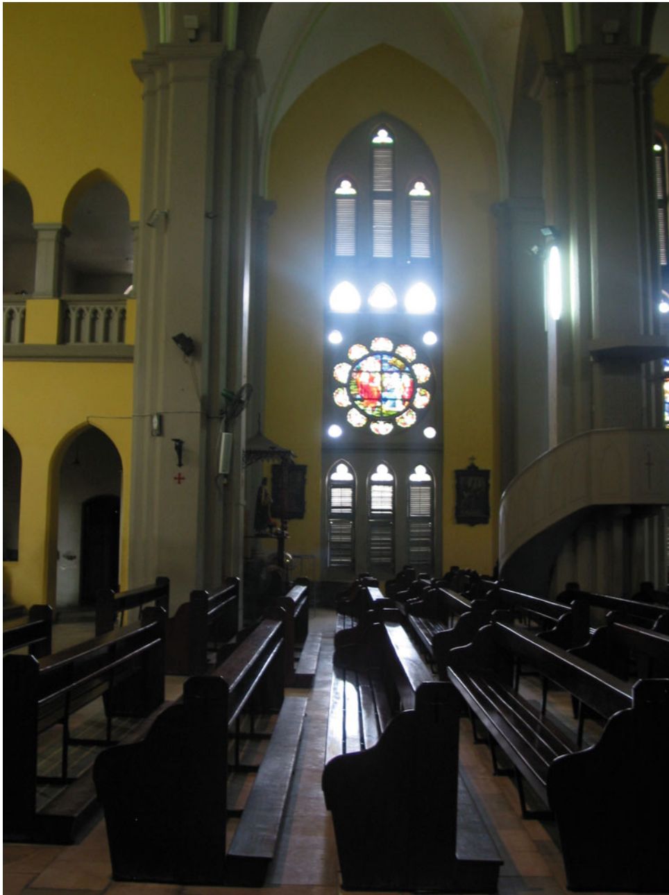
16.7 The new fenestration of St. Joseph's Cathedral with the lowered ventilation openings (see also p. 328). Photograph Belinda van Buiten
